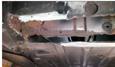
Left corner you see the new rocker panel attached with glue and one screw, but it looked ok from the top.
