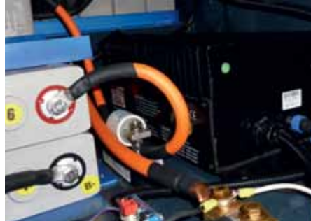
AC-DC charger, fuse, batteries in rear hold
