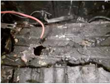
Rostskador under batteriet.
